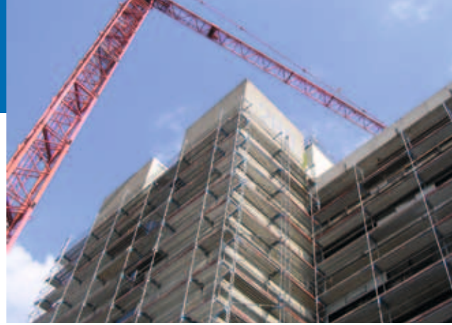
The major renovation work currently in progress at the DKFZ should be completed in 2010.
